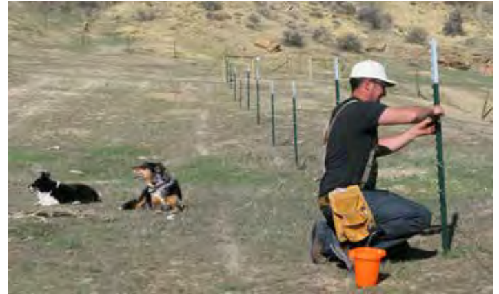
Nate Schmeiser puts the finishing touches on the Buyok fencing project on March 31 st .
