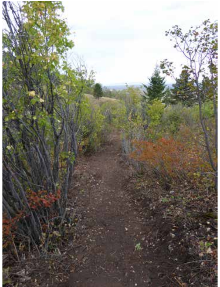
A completed section of trail on September 19 th . The trail’s appearance will improve significantly as understory plants fill-in and native re-seeding takes place, which is scheduled for November 2015.
